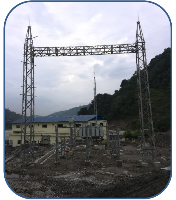
Power House Switchyard
