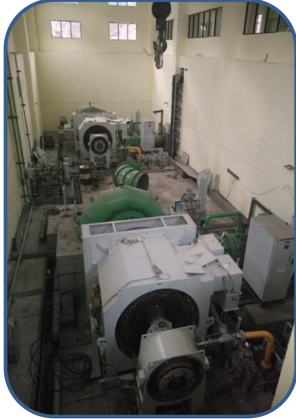
Power House Machine Hall
