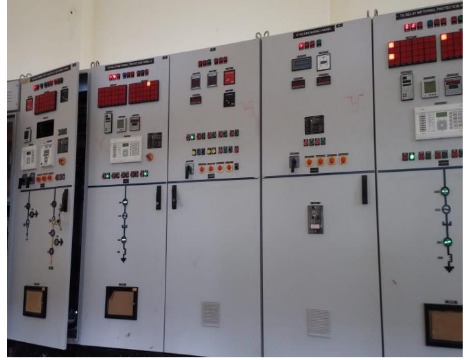
Power House Control Room Panel Testing on Progress
