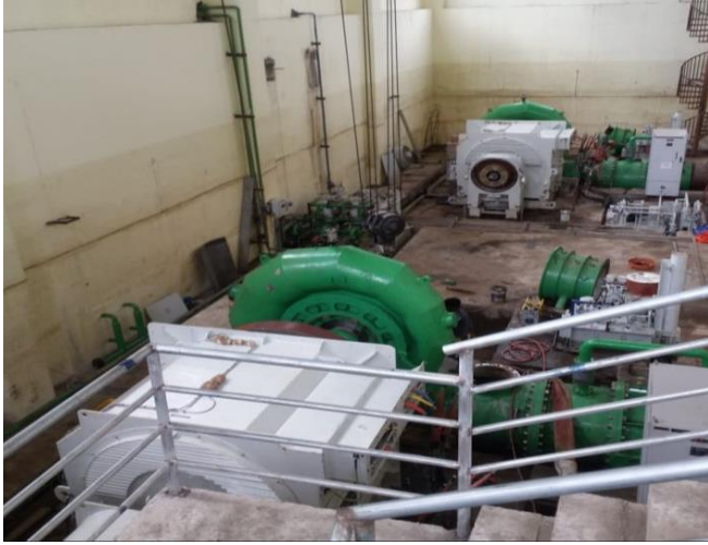
Power House Machine Hall
