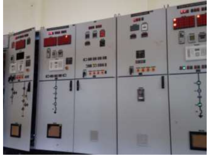
Power House Control Room Panel Testing on Progress
